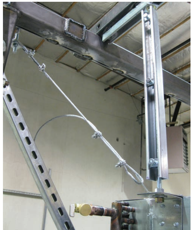
FIGURE 6 – UNISTRUT USED TO STRENGTHEN THE ROD
