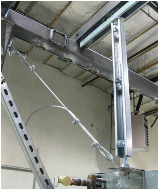
FIGURE 8 – UNISTRUT USED TO STRENGTHEN THE ROD
